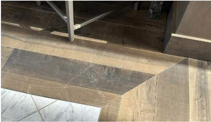
Scratches on wood flooring at bar area
